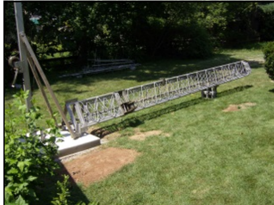
And on July 24th the tower was set onto the base along with the tiltover crane and winch.
