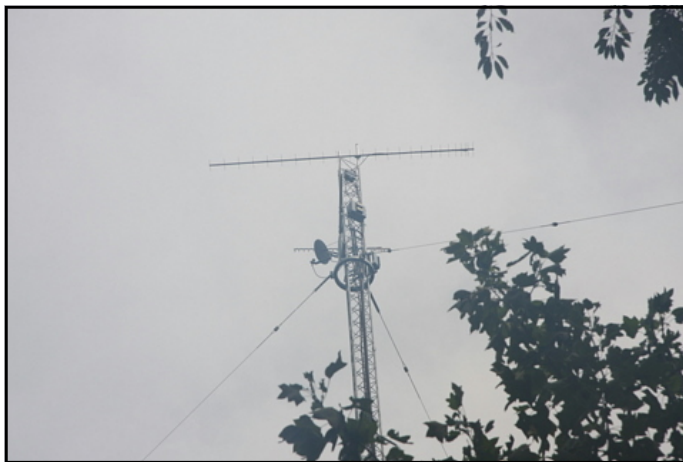
Phil's nearly complete rotating tower with some antennas already mounted
