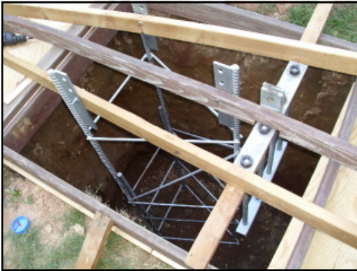
It takes a lot of steel and cement to hold up a free standing tower
