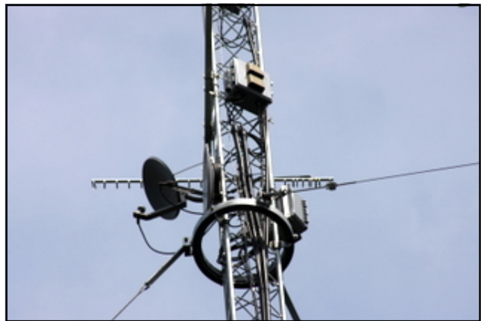
1296 Electronics and Antenna and 10 GHz dish, just above the top tower ring
